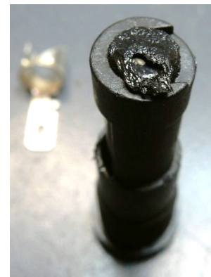
Figure 3: Localized melting of fuse holder
