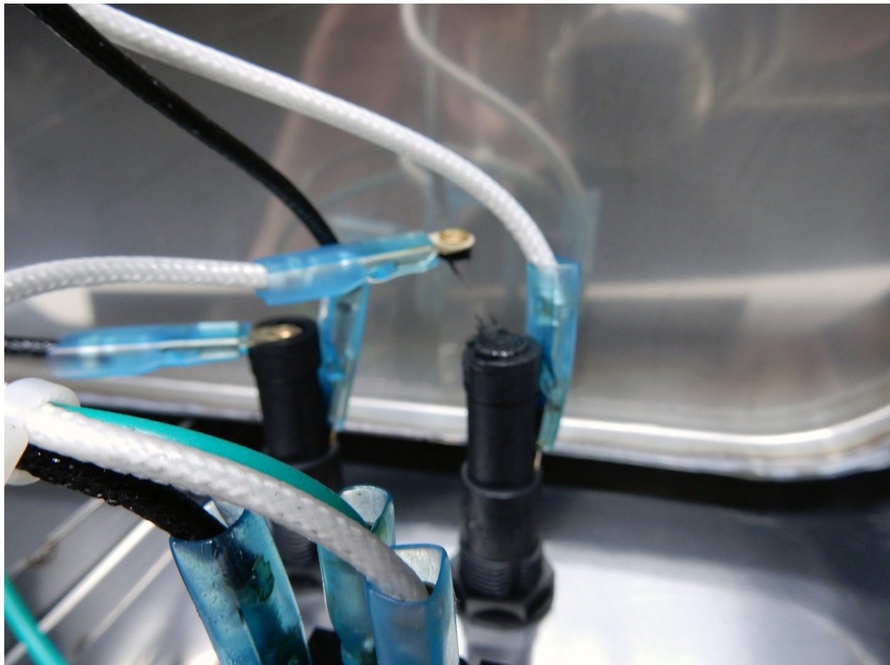
Figure 1: Terminal detached from neutral fuse holder
