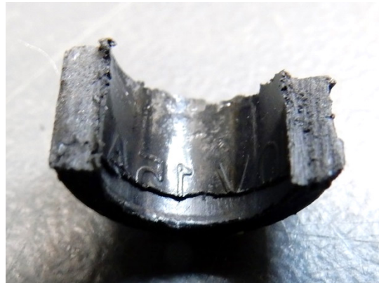
Figure 2: Embossed markings of fuse cap transferred to plastic of fuse holder (mirrored "0V 15A")
